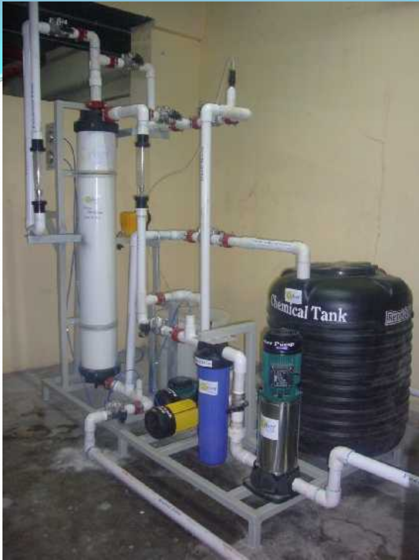
5M3/HR ULTRAFILTRATION (Sewage Recycling Plant)
